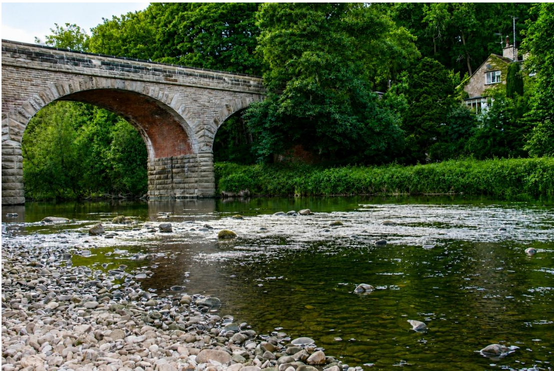
Figure 6 The bridge prior to its repair
