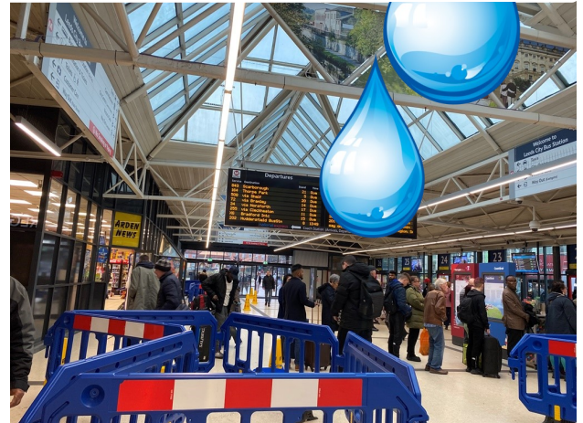
Their flagship Bus Station has been leaking for years. How much money is spent on this every year without it being fixed?
